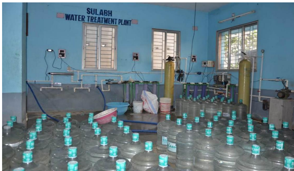
Figure 2: Rural Water treatment Plant in Madhusudankati SKUS Ltd
